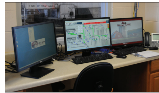
The mill is controlled by Beta Raven automation software.
