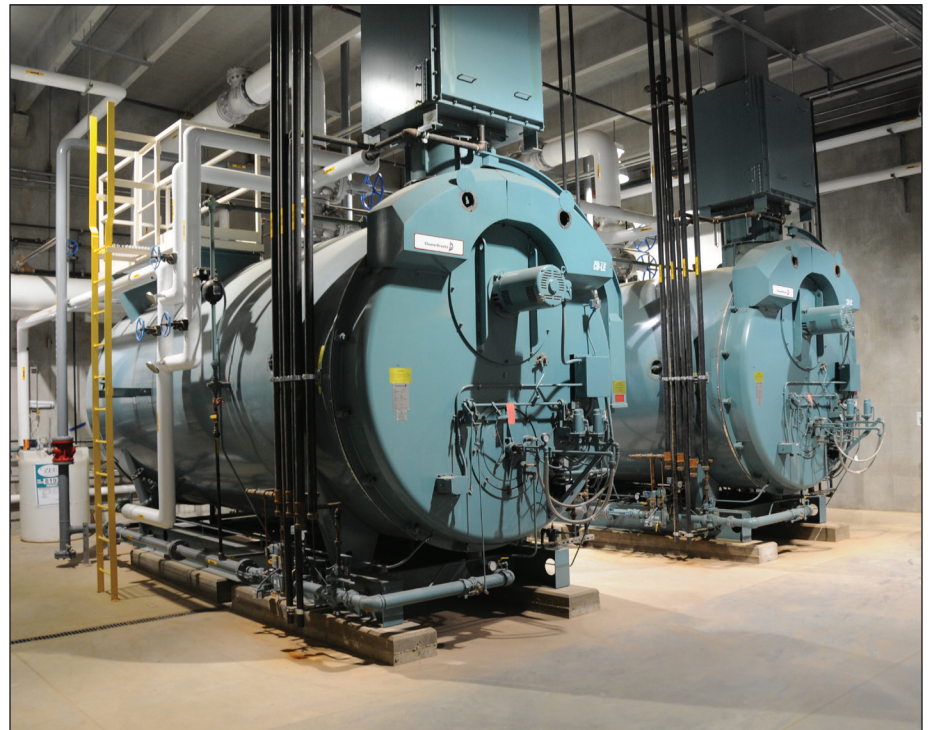
Two Cleaver-Brooks 600-hp boilers supply steam for conditioning during the pelleting process.
