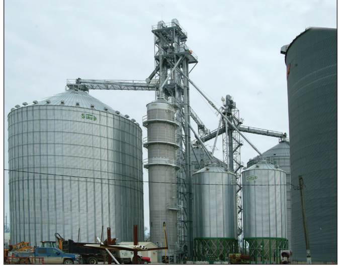
Ground-level view of new construction, from left: 515,000-bushel Sukup steel tank; 4,700-bph Sukup tower dryer; Tri-Co support tower encasing three Schlagel legs and a Schlagel Swing-Set distributor; and to 30,000-bushel Sukup wet tanks. Photo by Jerry Perkins.
