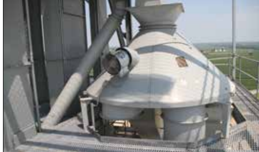
One of the three Schlagel electric rotary distributors.
