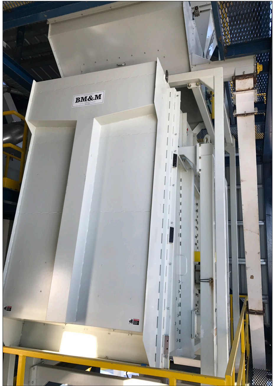
BM&M Rotary Super-Flo cleaner is part of a cleaning house operation designed to clean wheat to Canadian export standards at 240 mtph (8,800 bph).
