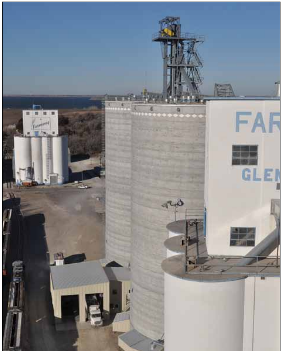
Another view of the expansion project at Glen Elder from the roof of the main concrete house, with new construction in the center of the photo.
