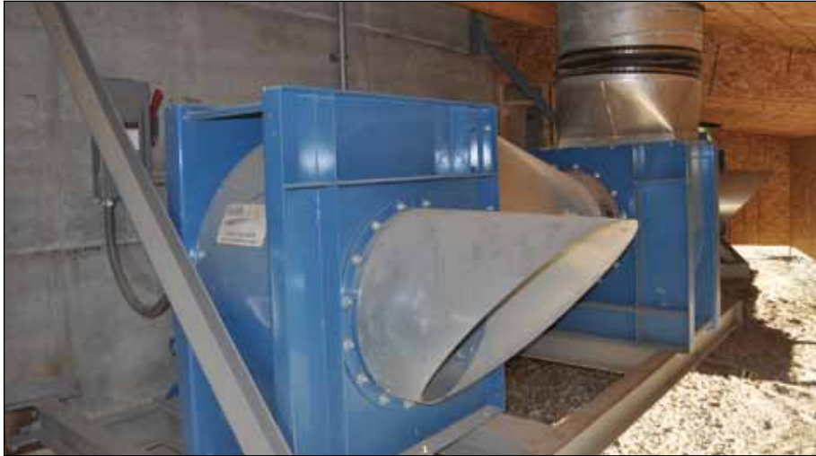
The two photos above depict a sound-muffling enclosure designed by AIRLANCO to reduce noise levels for nearby residents.
