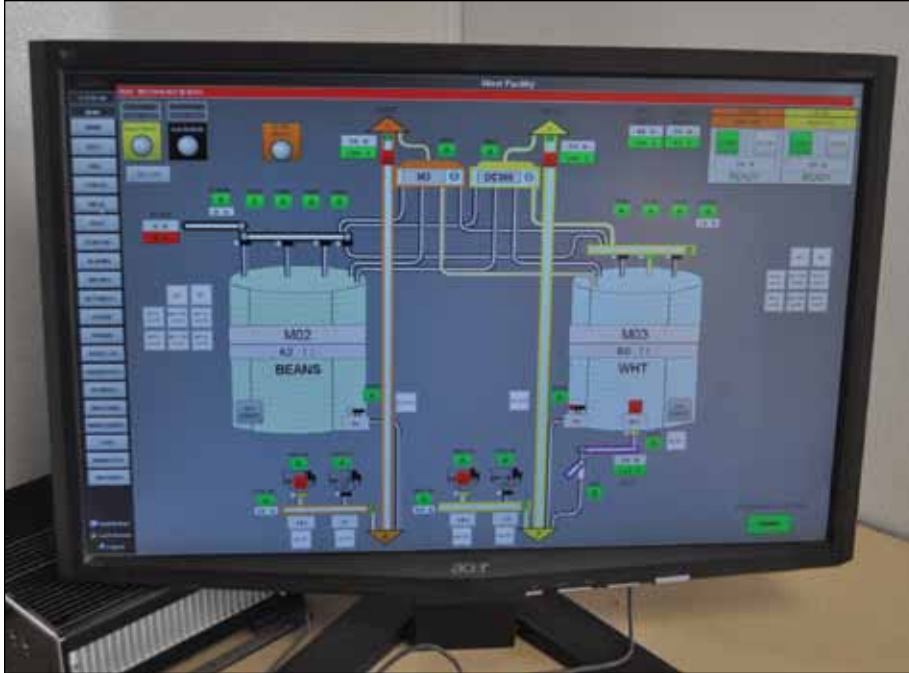
One of many screens available to elevator operators via a KASA control system shows the contents of two new jumpform concrete tanks and status of equipment serving those tanks. Additional photos by Ed Zdrojewski.
