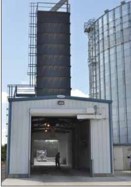
New receiving pit features a dump-through truck scale that reaches a 20,000-bph receiving leg.
