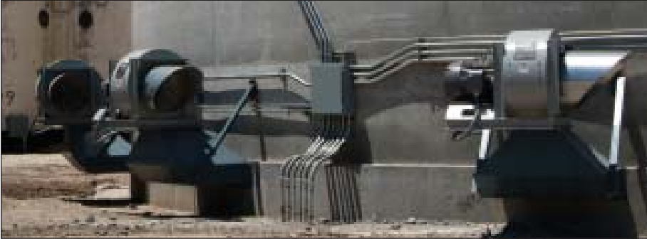
New tanks are outfitted with half a dozen Rolfs@Boone 60-hp centrifugal fans supplying 1/6 cfm per bushel worth of aeration.
